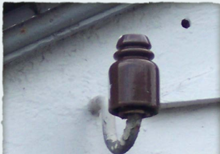
Brown terminator in situ on house
